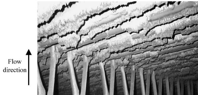
Fig. 2. Photograph of deposit formation in a lignite utility boiler (PPC of Greece).
